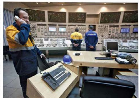
A company official inside one of Kyivenergo's thermal energy plants that belongs to Rinat Akhmetov, the nation's richest billionaire, speaks on a phone. The city's municipal heating company owes more than $500 million to Naftogaz for unpaid gas deliveries.
