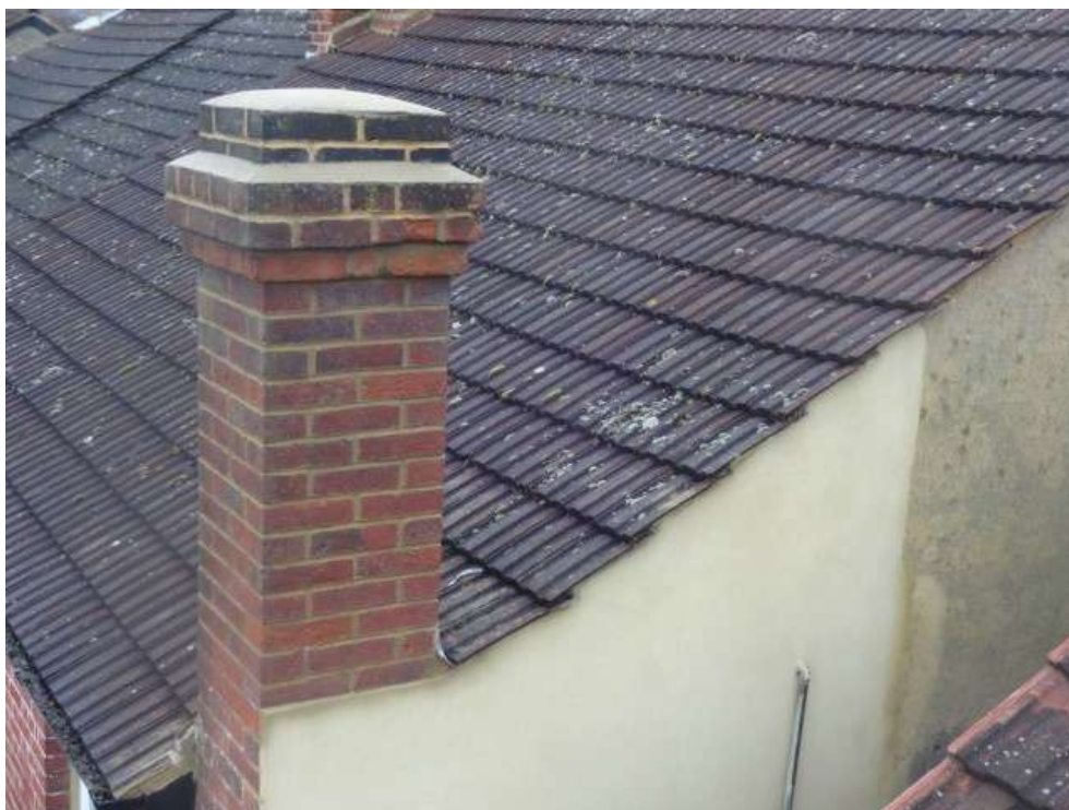
Front bedroom chimney capped stack Change position
