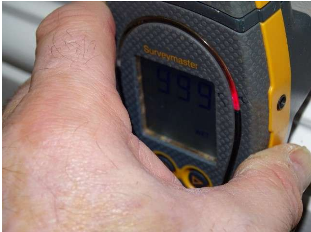
Dampness to front wall of sitting room
