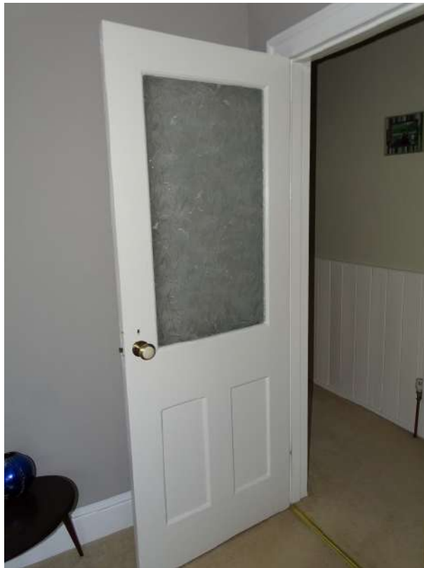
Non safety glass to sitting room door
