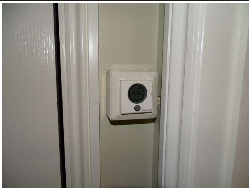
Room stat to underfloor electric heating
