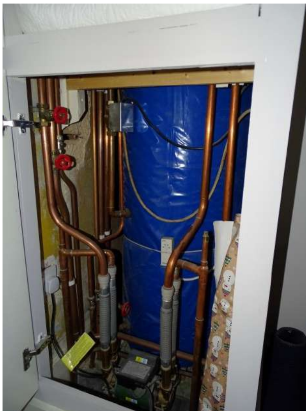
Hot water cylinder with back up immersion heater
