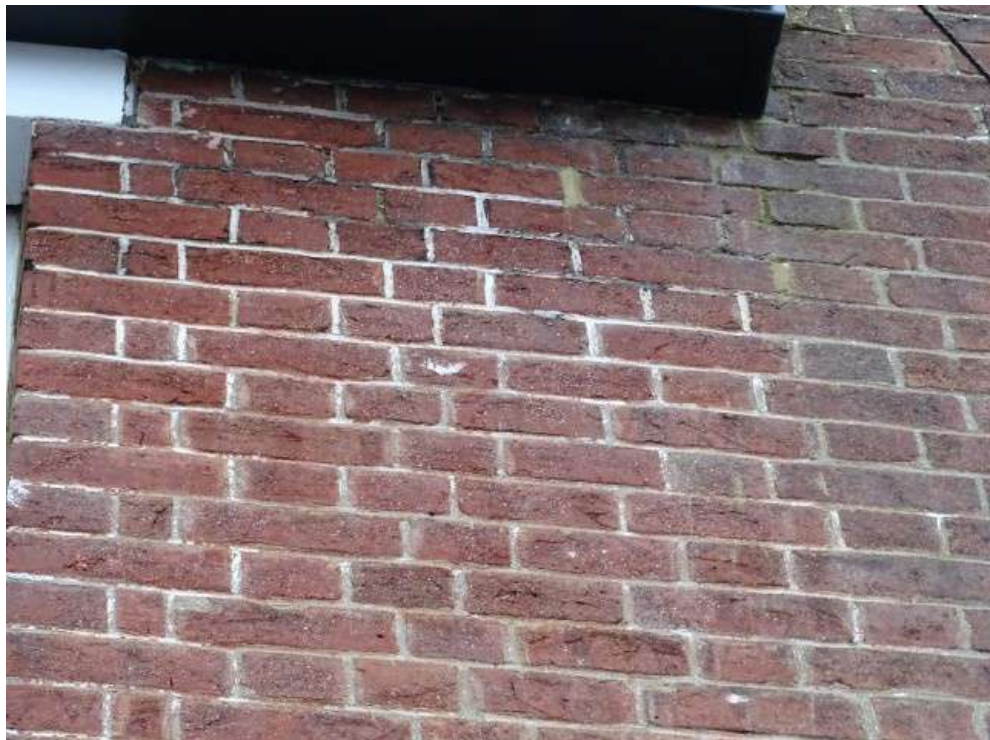
Re-pointing required to right hand side of bedroom 3 window
