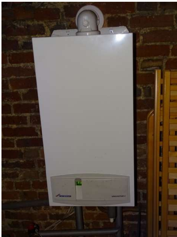
Gas boiler in loft
