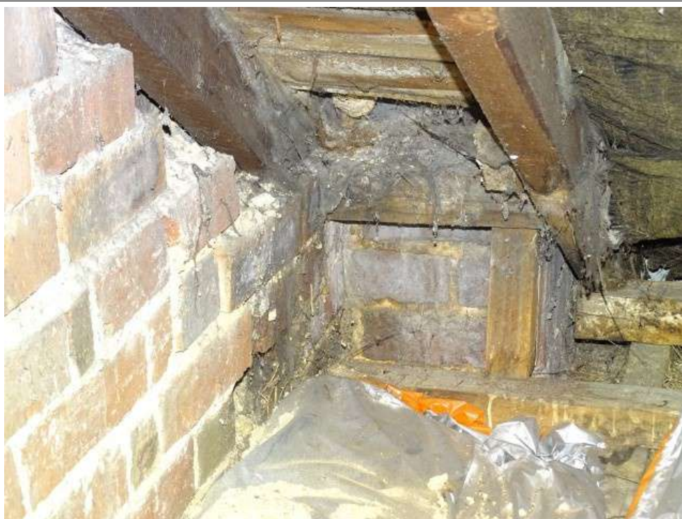
Chimney stack from small front bedroom showing dropped sarking felt
