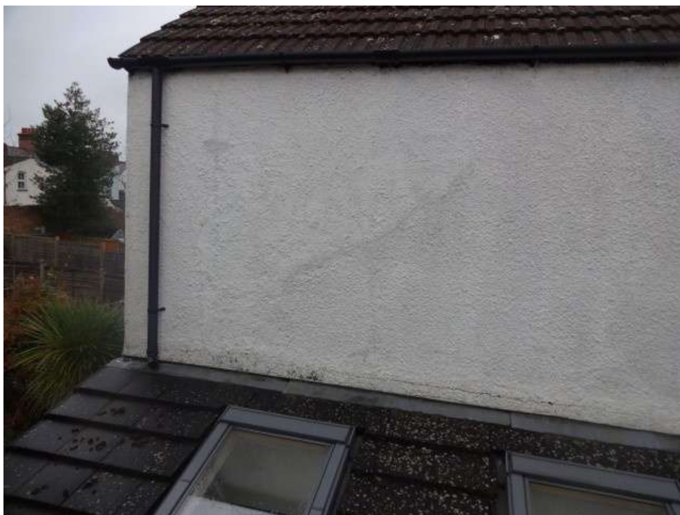
Cracked render to bedroom 4
