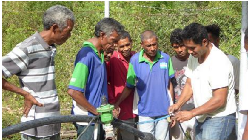
Figure 3-40: BESIK pump technician installing a new pump at Rau Moko in Lautem municipality (BESIK, 2015)
