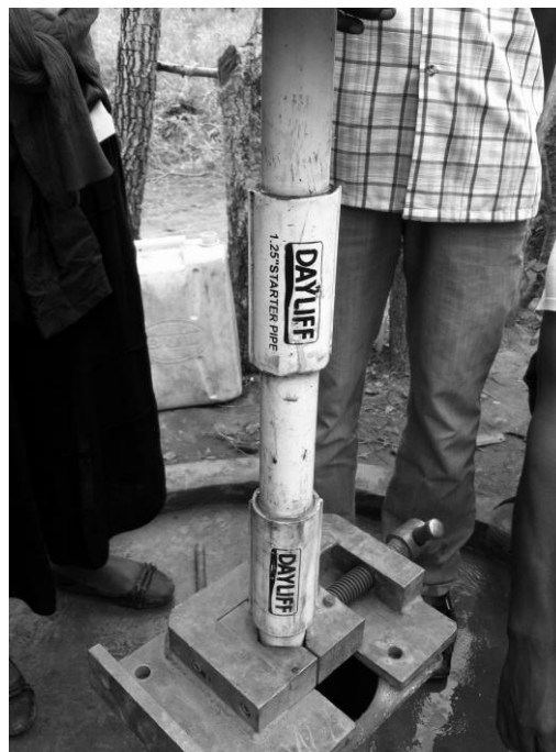
Figure 6. 1¼" PVC riser pipe fitted to an India MkII pump at Angodingod
