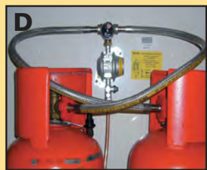
Picture shows a Truma regulator upgraded to a manual changeover with a 01-1630 and using two propane 0.75 meter Stainless hoses. Note how the hoses cross preventing unnecessary kinking and twisting.
