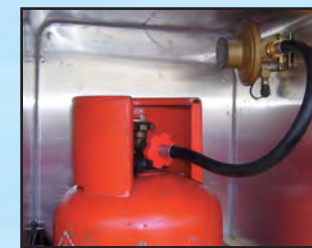
A single 0.45m EasyFit rubber hose system fitted to a Nova Comet 30mbar system.
