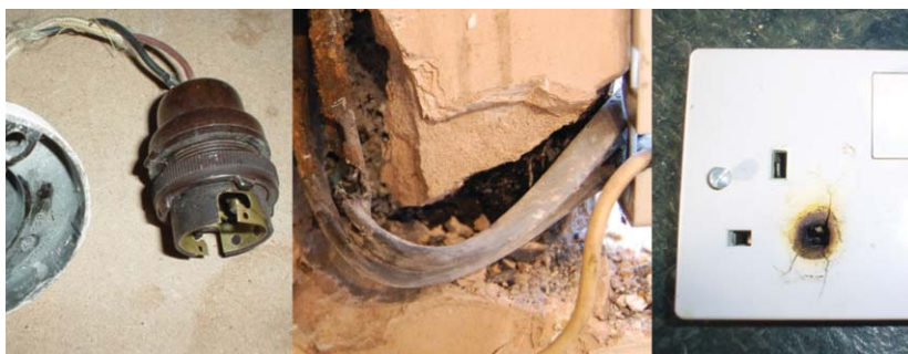
▲ Typical examples of potentially dangerous electrical installations
