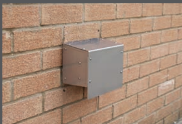
Remote Control Air Intake Box
