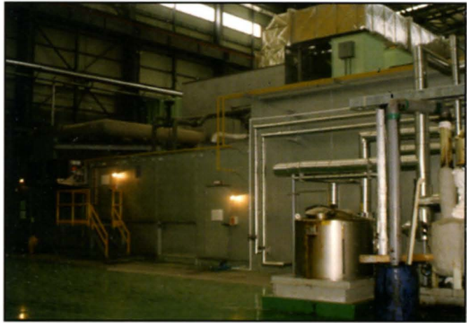
Hyundai Power Company, Korea Daesan, Siemens SGT6 3000E
