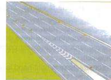
Road traffic markings and reflective road studs
