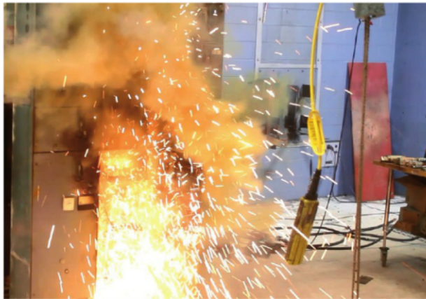
The next edition of IEEE 1584 will provide more options for modeling equipment
