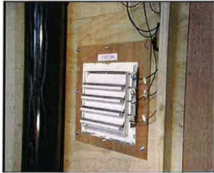
Photo of AES300 pressure vent with risk pressure at 790 Pascals. Vent in maximum open position.
