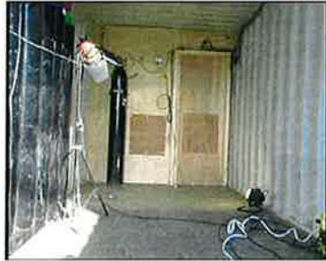
Photo of IG55 discharge with no venting risk pressure reached 1700 Pa
