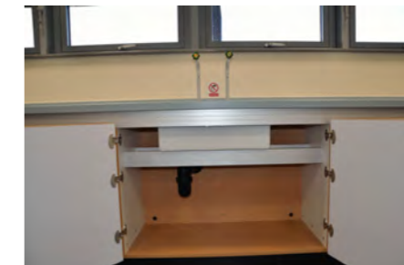
Re-enforced sink supports & complete back panel service Void protection for all units Inc. sinks units.
