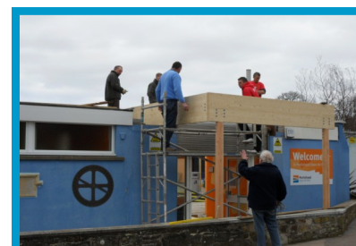
The new entrance takes shape—Stuart Hamer of Glulam, Paul Richards and James Hailwood of Richwood Construction , ably assisted by volunteers
