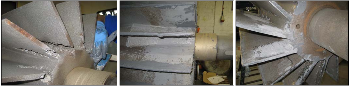
Suction impeller after grit blast - after application of 1311 - after being ground to profile
