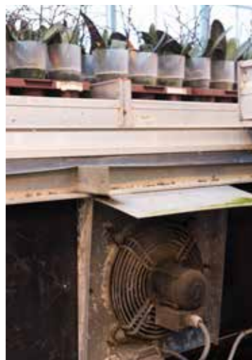
Floor-based convectors, over the full length of the greenhouse and in between the bays, are covered with a grid. Fans draw in air through the grids, direct it along the tubes before distributing air masses equally under the rolling benches.
