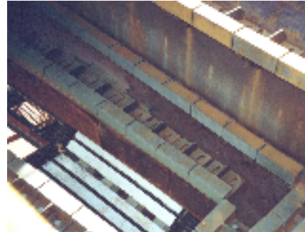
BELOW: Rock-boxed product screen bottom-deck oversized chute at
