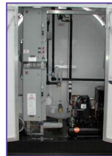
Electrical panels inside control cabinet for refrigeration system and optional pressure build vaporizer
