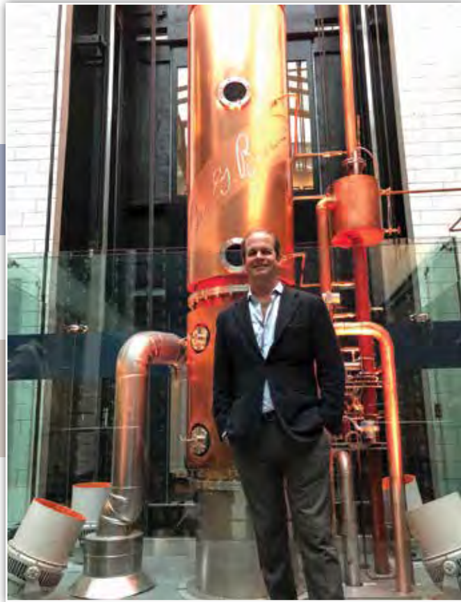
Old Forester President Campbell Brown stands in front of the 44-foot-tall copper column still at the new Old Forester Distilling Co. located on Whiskey Row in downtown Louisville.
