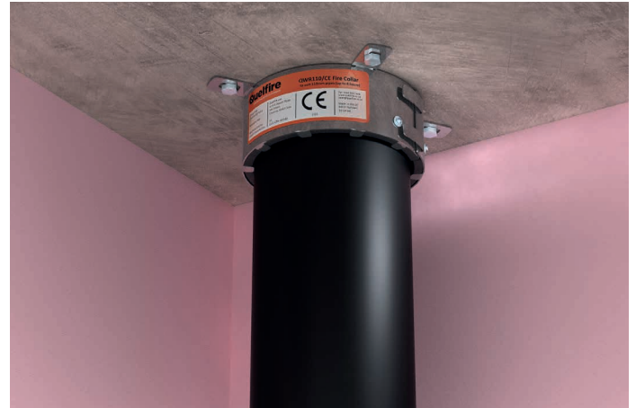
QWR CE Marked Fire Collar installed on concrete floor
