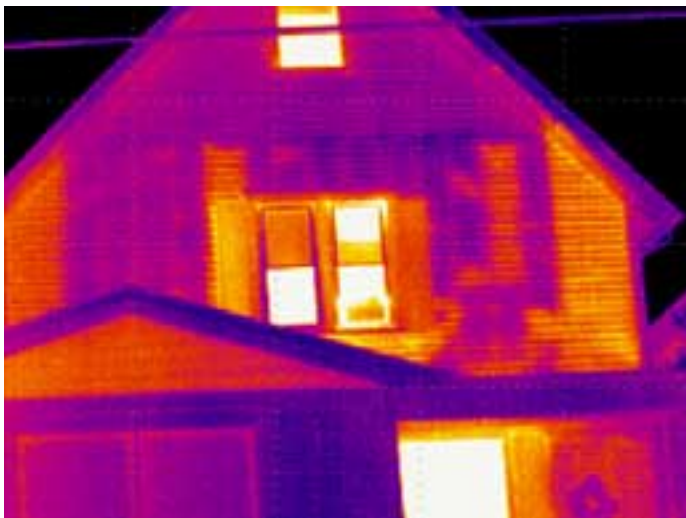
This home clearly has missing insulation in the front wall and, on either side, a poor definition of the thermal boundary. Over the life of the building, these problems will cost thousands of dollars and result in a drafty, uncomfortable house, perhaps with serious moisture problems.
