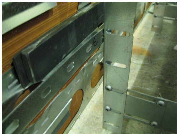
Photo 8. Start of failure.
