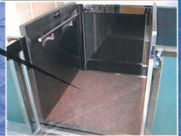
● LIFTING PLATFORM IN AN OFFICE PREMISE
