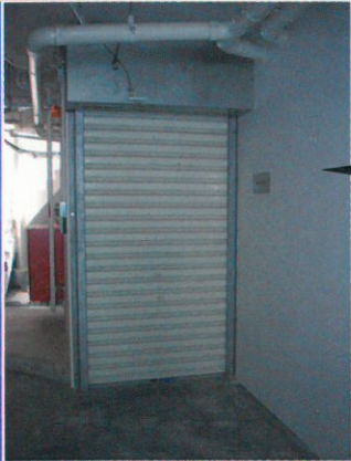
● BIN LIFT AT A CONDOMINIUM
