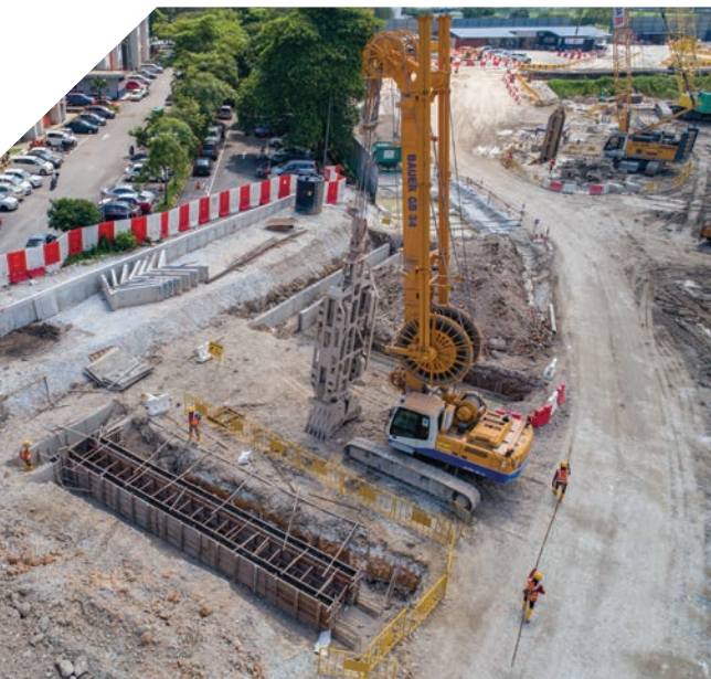
Diaphragm Wall for the intervention shaft and the crossover of Mass Rapid Transit 2 project, Malaysia
