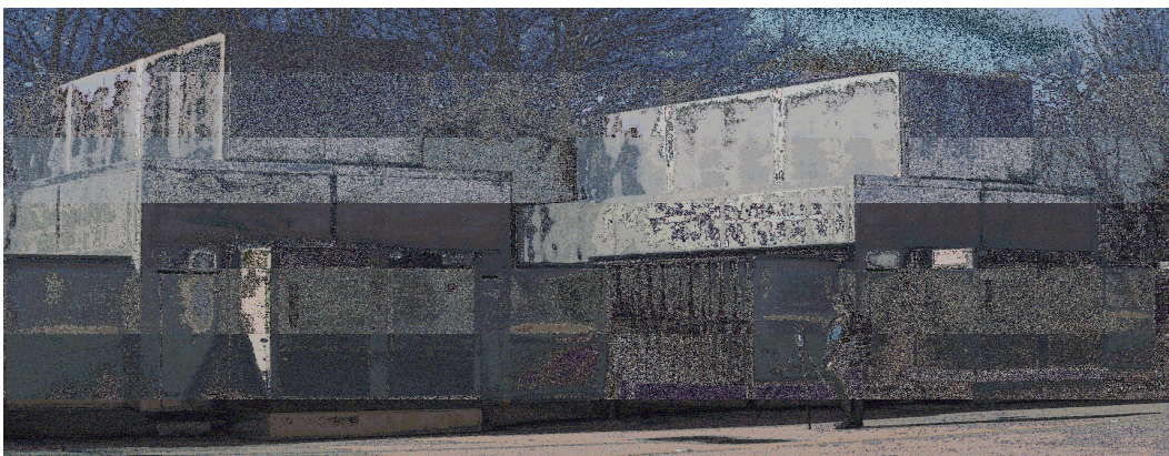
Photograph showing two air-cooled water chillers with full attenuation packages.
