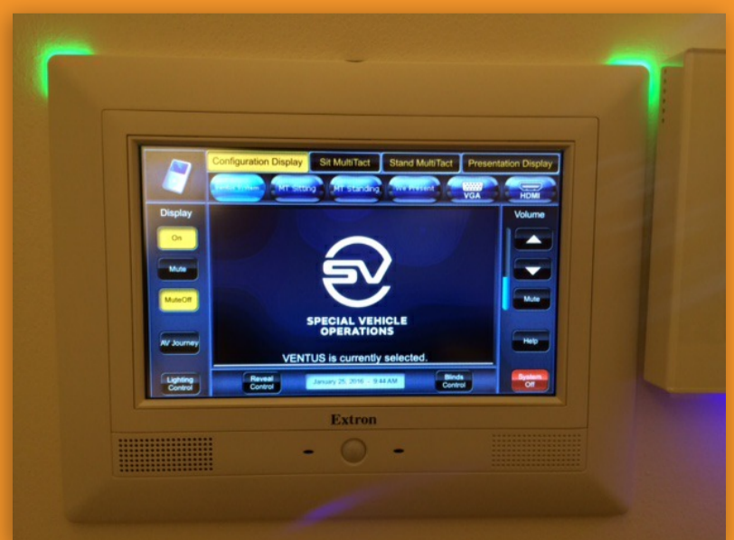
Main Control Panel
