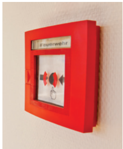
Fire Safety Systems
