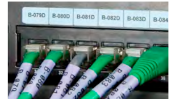
Patch Panel Labels
