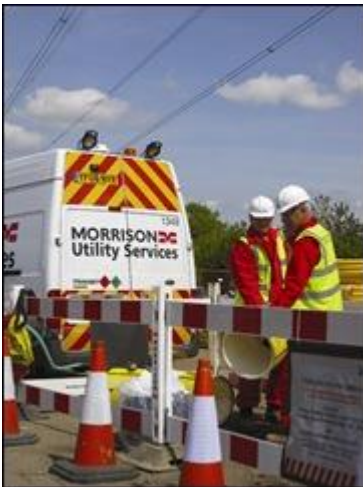
Some sites are just temporary so a service provider has to have flexibility and understanding
