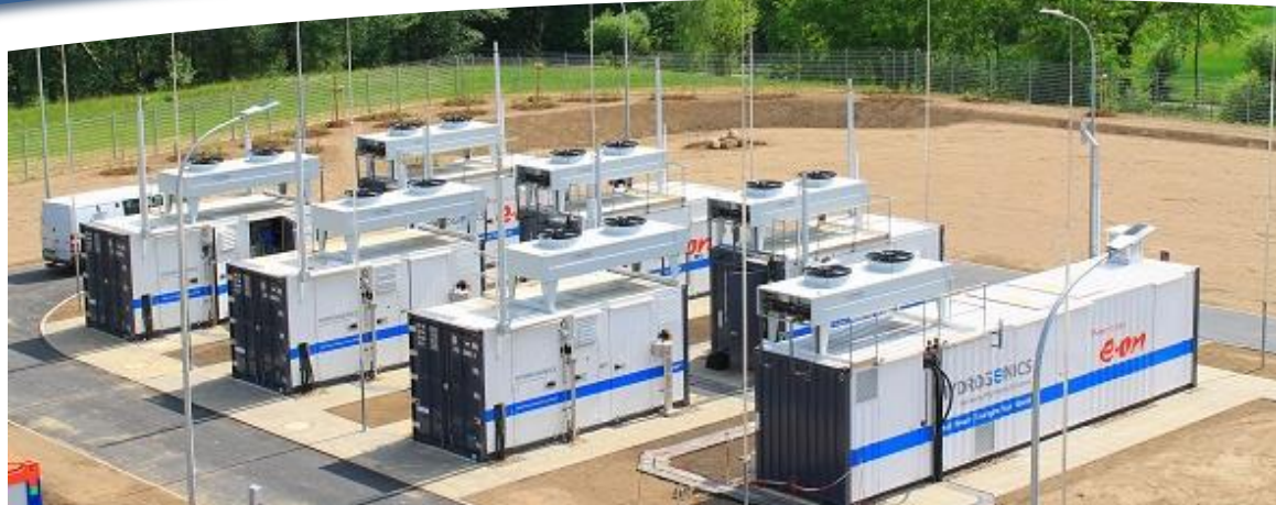
Power-to-Gas plant in Falkenhagen, Germany
