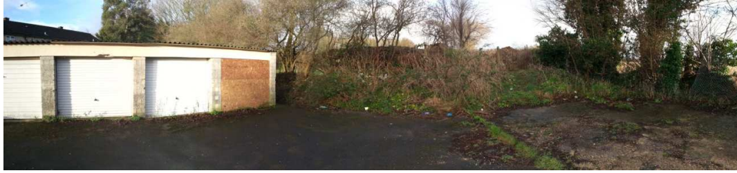
Image 06: A wide angle shot of the larger garage block adjacent to an access path and trees to the north of Northcroft Road properties.
