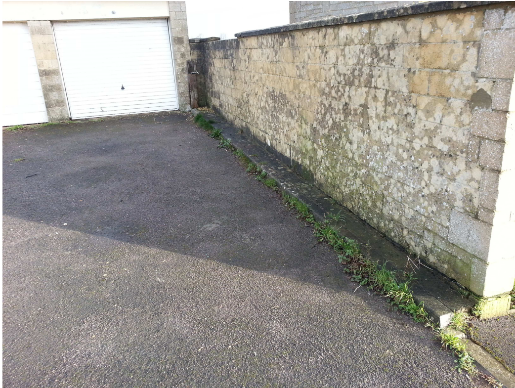
Image 02: Pivoting to the left, we see here the boundary wall between the first garage block on the left, and the GreenSquare block of flats to the right behind the wall.
