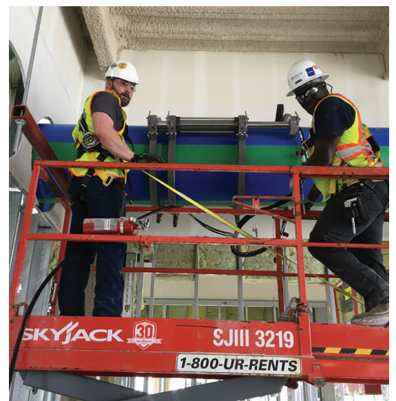
Kirlin's installation team heat-fusing large-diameter Aquatherm pipe using a prototype McElroy Acrobat™ 630 at the Seminole Hard Rock Hotel & Casino.
