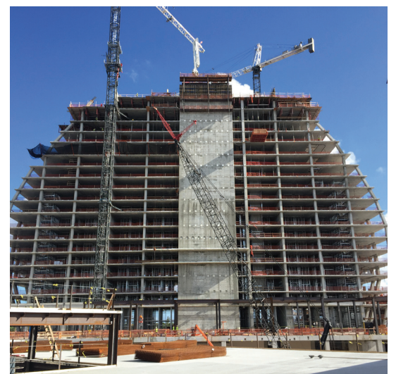
The signature guitar-shaped main building take shape at the Seminole Hard Rock Hotel & Casino in Miami.
