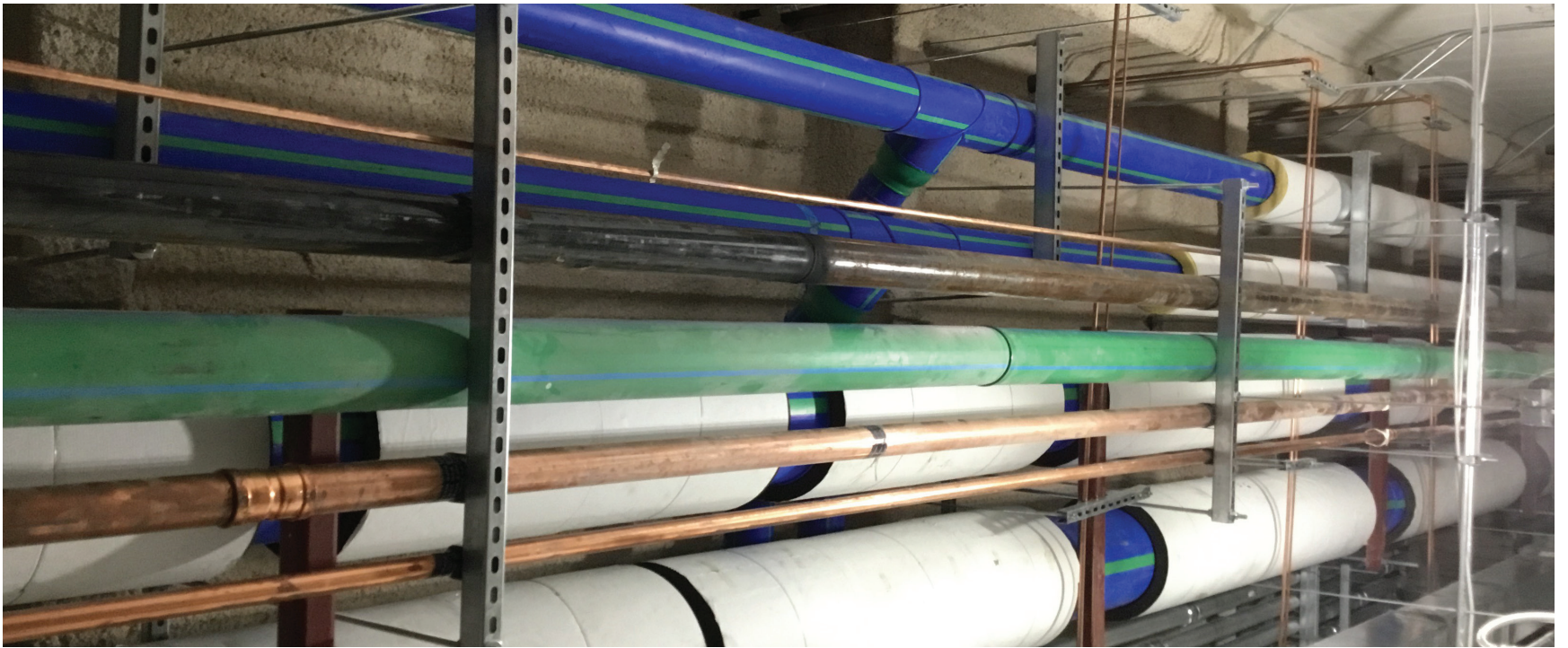
Aquatherm pipe sizes ranging from 3/4-in. to 24-in. installed at the Seminole Hard Rock Hotel & Casino.
