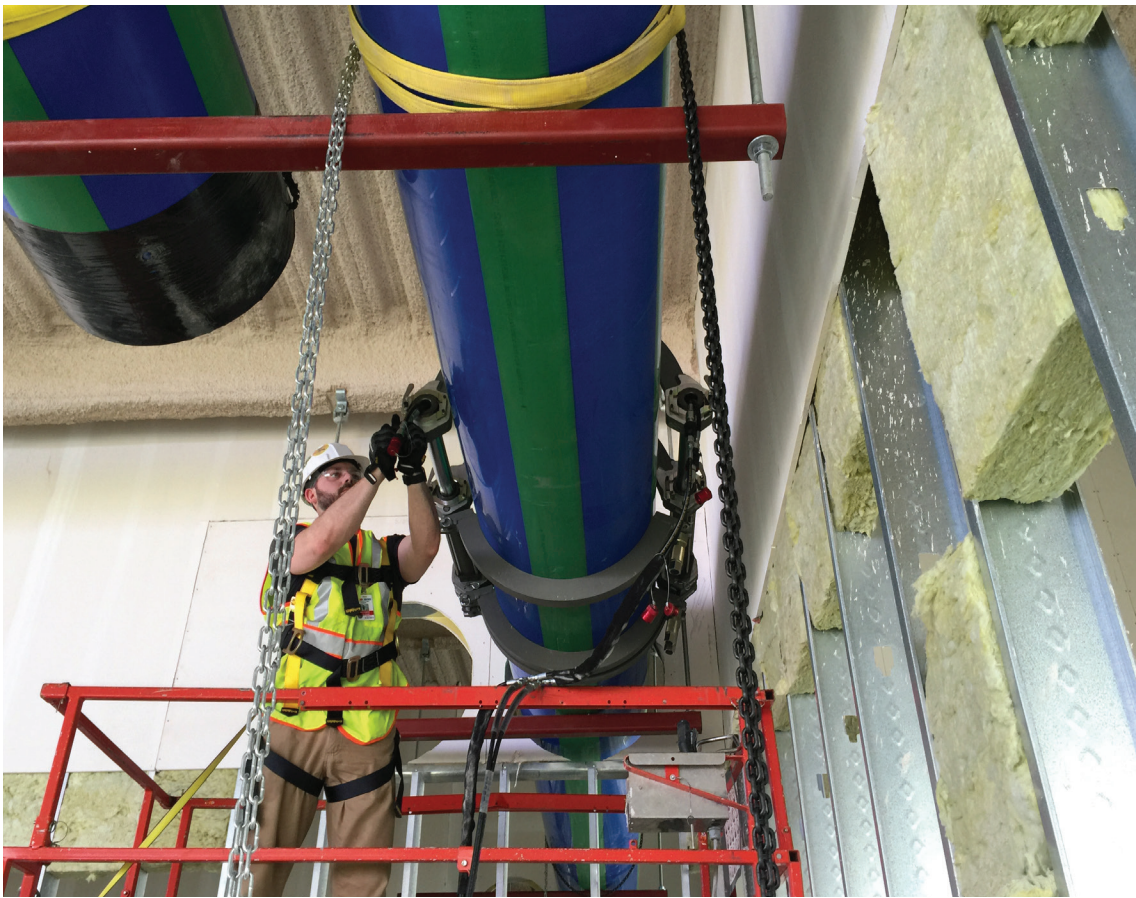
Trying to weld steel pipe overhead, on a scissor lift, in tight spaces, could be very difficult. But Aquatherm PP-R pipe and McElroy fusion equipment changed the game at this hotel and casino.
