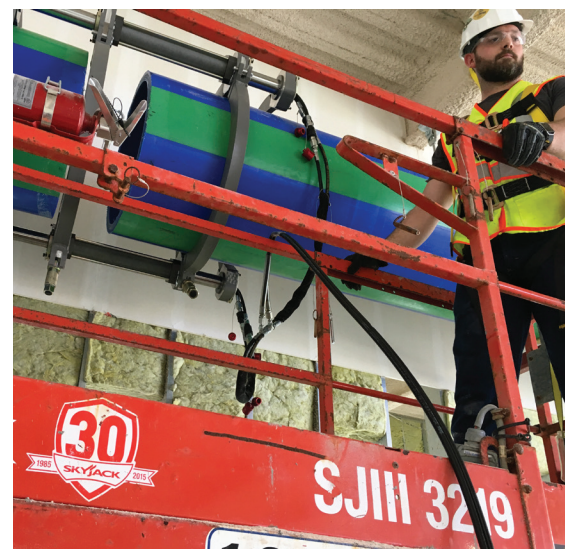
Trying to weld large diameter pipe overhead in tight spaces can be difficult and time-consuming, but the decision to use heat-fused Aquatherm pipe helped keep this project on schedule.
