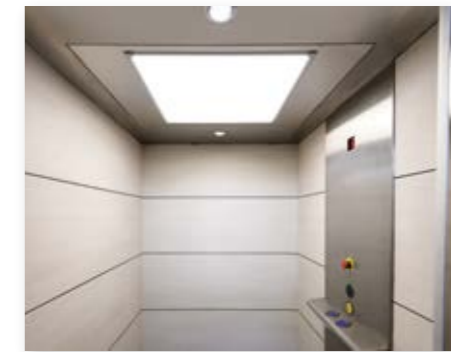
8 LIGHTING LEDs panel
