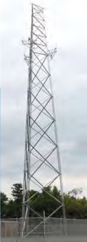
Cell Tower, — Groveton, NH
