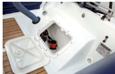
Bilge and pump access
