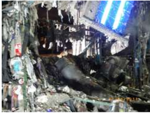
Damage on platform looking out onto Sheffield Road
