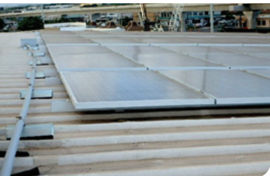
Bending conduit on the roof. This can damage the wires and lead to problems.
