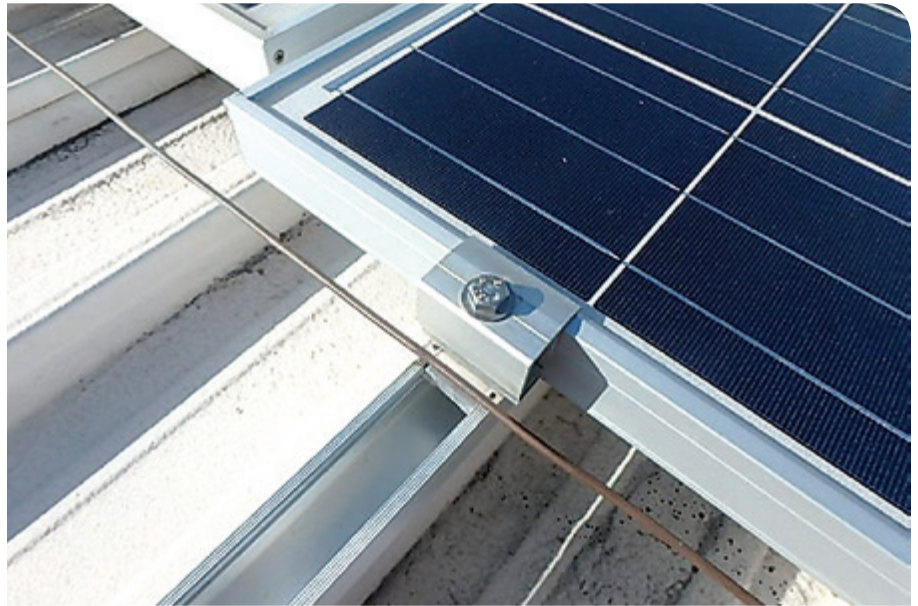
This end clamp is properly installed, but the grounding clip is not being used as intended.
