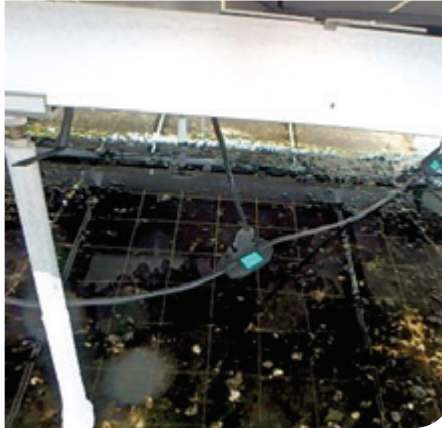
Hanging wires that sit on the roof deck are subject to sitting in ponding water.
