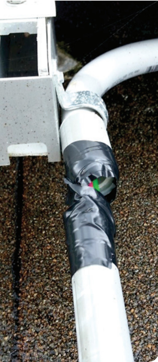
Damaged piping that has been "fixed" with electrical tape, and is now exposing wires to damage and the elements.
