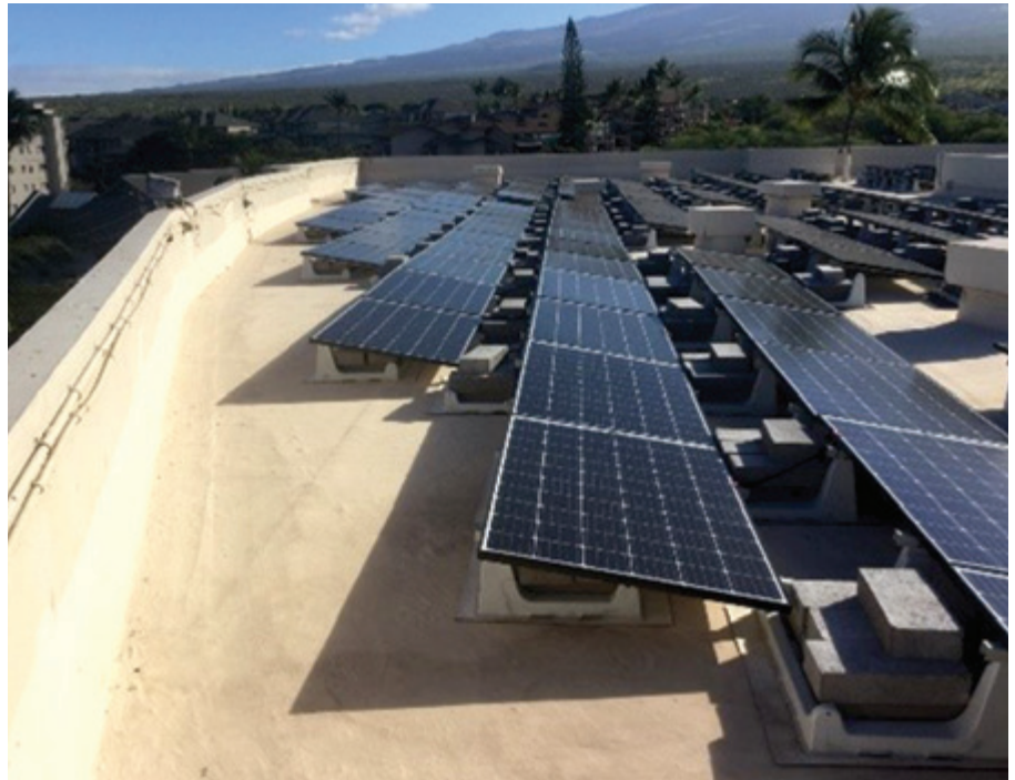
Ballasted PV System with slip sheets beneath ballast pans
