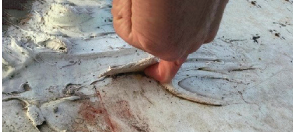
Poorly sealed flashing at PV standoff
