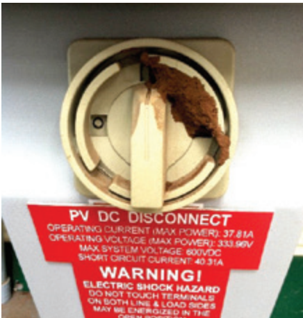
Proper labeling on the disconnect that displays system production numbers. This handle was home to a happy mud wasp.
