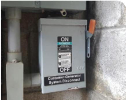
Labeled system disconnect
