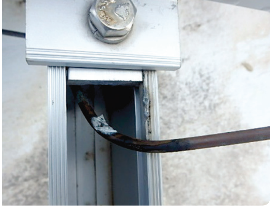
This damaged wire caused a short in the system, and has an arc mark on it. Luckily, that was all that happened due to the wire not being properly secured and protected. A burn mark can be seen on the rail
