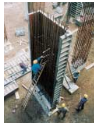
A 6.60-m high column formwork with MANTO panels 330—and only one panel joint at such a dizzy height!
