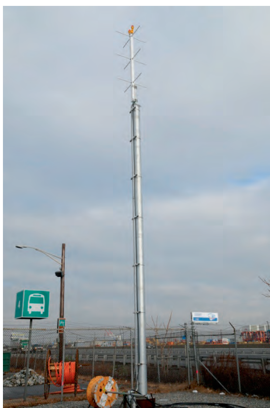
Figure 1. Newark VDB Antenna Next to a Multi-Lane Freeway
