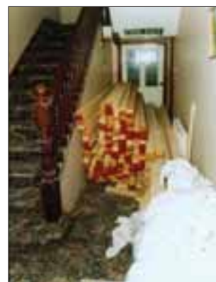
Figure 9: A blocked corridor with incorrect signage
