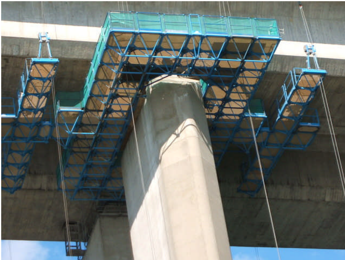
The ALPS Steel Truss Frame Access & Lifting Platform shown in place at bearing level.
