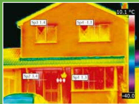
The warmest areas seen here in red show where heat is being lost from the building.
