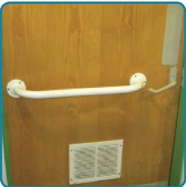
A light action lever lock on the inside of this toilet is easy to use and changes the occupied / vacant indicator on the outside
