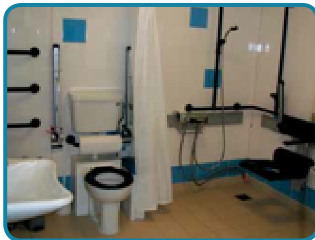
The CP facility at Ken Martin Leisure Centre in Nottingham includes a shower seat with a backrest and drop-down arm supports
