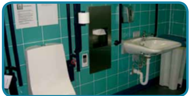
The fittings at the CP facility at City Hall, London, contrast visually with their background
