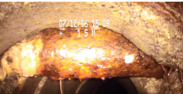
CCTV inspection showed several areas of concern in the sewers, including sections where water lines passed right through the sewer.
