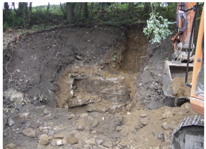
Figure 5. Excavation, revealing the former rock face beneath the existing ground surface representing the rear elevation of a former mill building that occupied the site.
