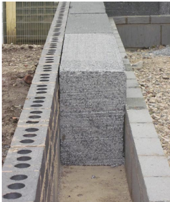
300mm closed cell EPS full-fill cavity wall insulation below DPC level, ready to be used as shuttering for the poured concrete floor.
