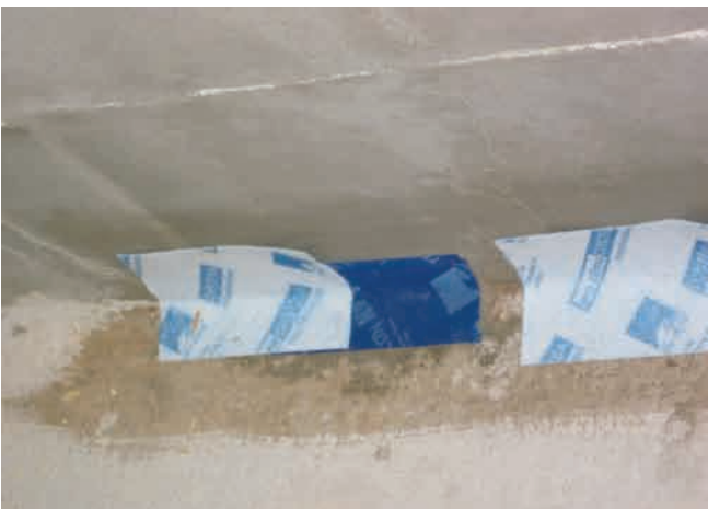
Top: neat tidy taping of window units to plywood window surround boxes. Centre: air tight parge coating behind all MVHR ducts against walls. Bottom: trial air tight taping experiments of damp plaster wall to damp concrete slab with primer base. Nothing much would stick without drying every thing out first. Cement parging was also carried out around all electrical cable runs and back boxes.
