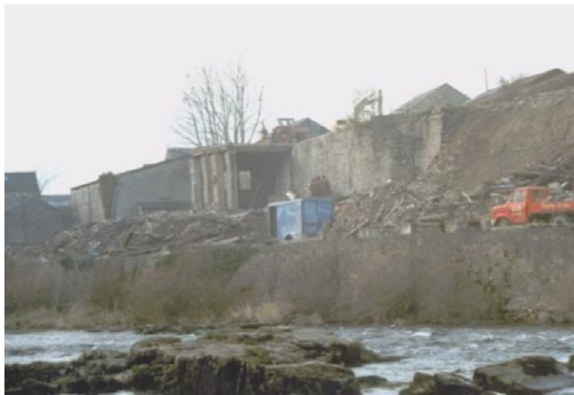
Figure 3. View of the site taken from the canoe videos showing the former mill during demolition showing the scale of the construction and the possible retaining walls that could be present on site
