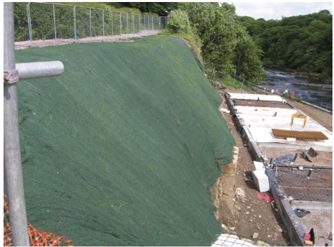
Figure 8. The finished slope with vegetation starting to grow through the anti-erosion matting.
