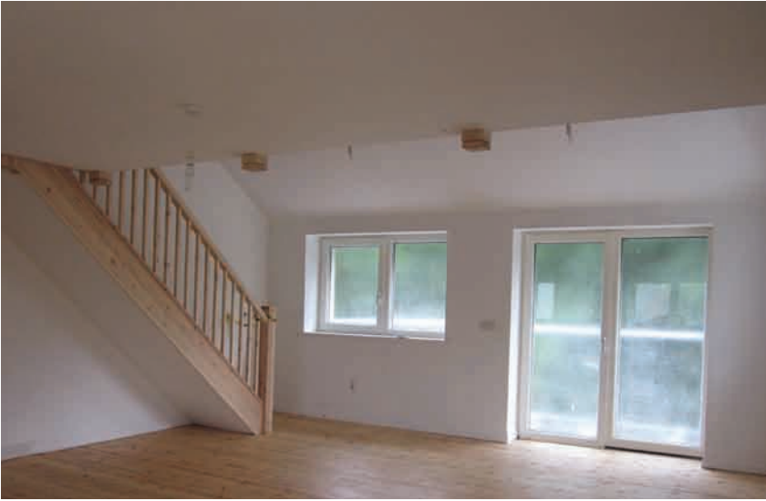
Inside view of one bed flat during air test (with staircase to mezzanine bed platform in the open cathedral roof space).
