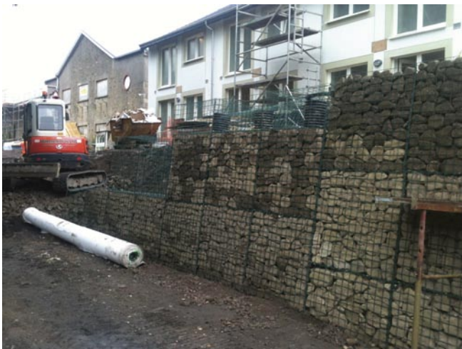
Figure 9. Gabion wall to the front of the terraces (with pipes built in to the top sections to receive the handrail uprights).
