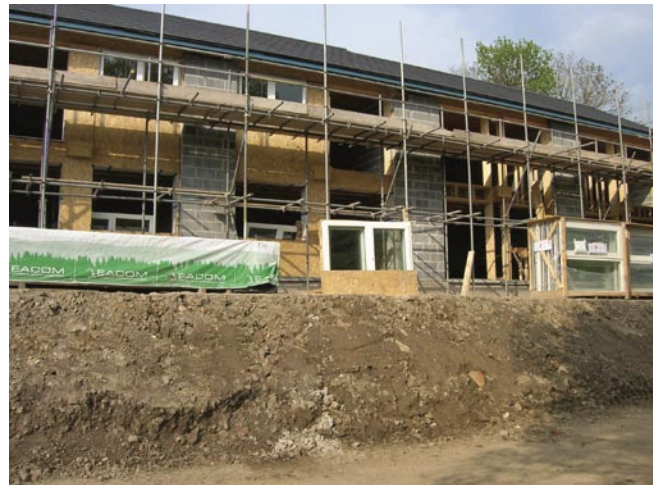
Figure 12. South elevation showing Kerto timber framed openings between Block work return walls at the end of party walls.
