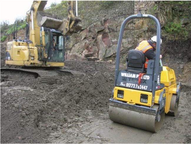
Figure 11. Compaction trials to determine the appropriate plant, number of passes and degree of vibration to compact the site-won clay up-fill material.
