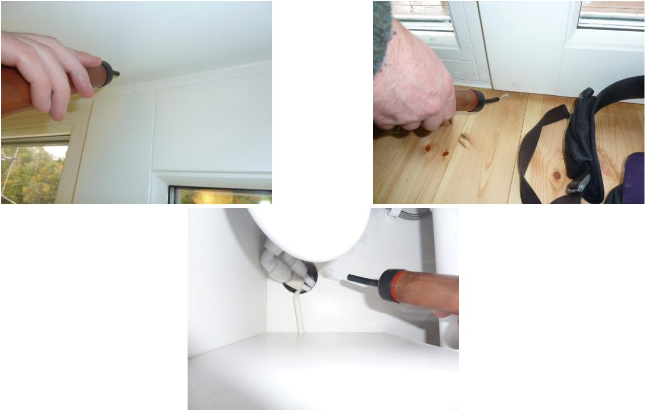
Figure 4 Small amounts of leakage at the top and bottom of the opening leaf of the patio door in the master bedroom and at service penetrations under the kitchen sink.
