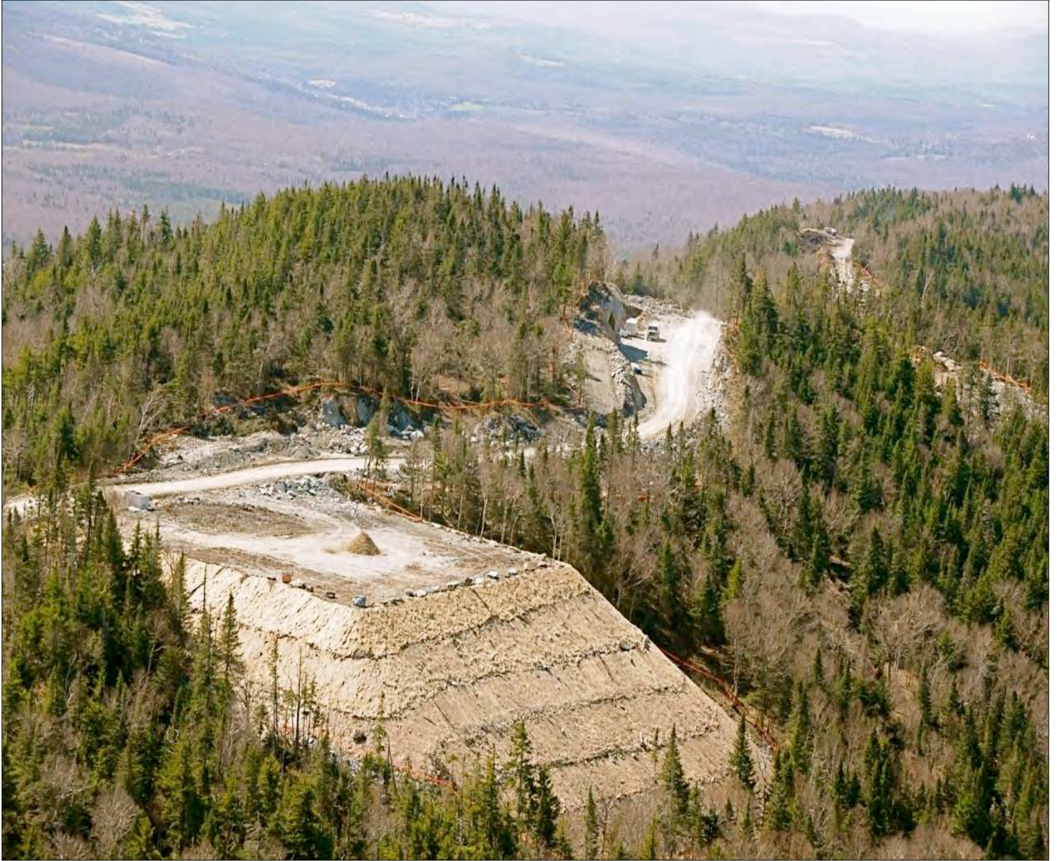
One of Twenty-One Wind Turbine Pads, Lowell Mountain, Vermont Photo by Steve Wright
