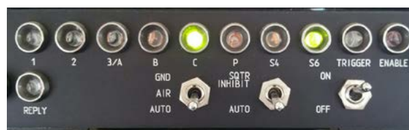
Figure 8 TPDS LED Panel
