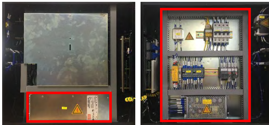
Figure 8.23 High voltage region inside I series control box.
