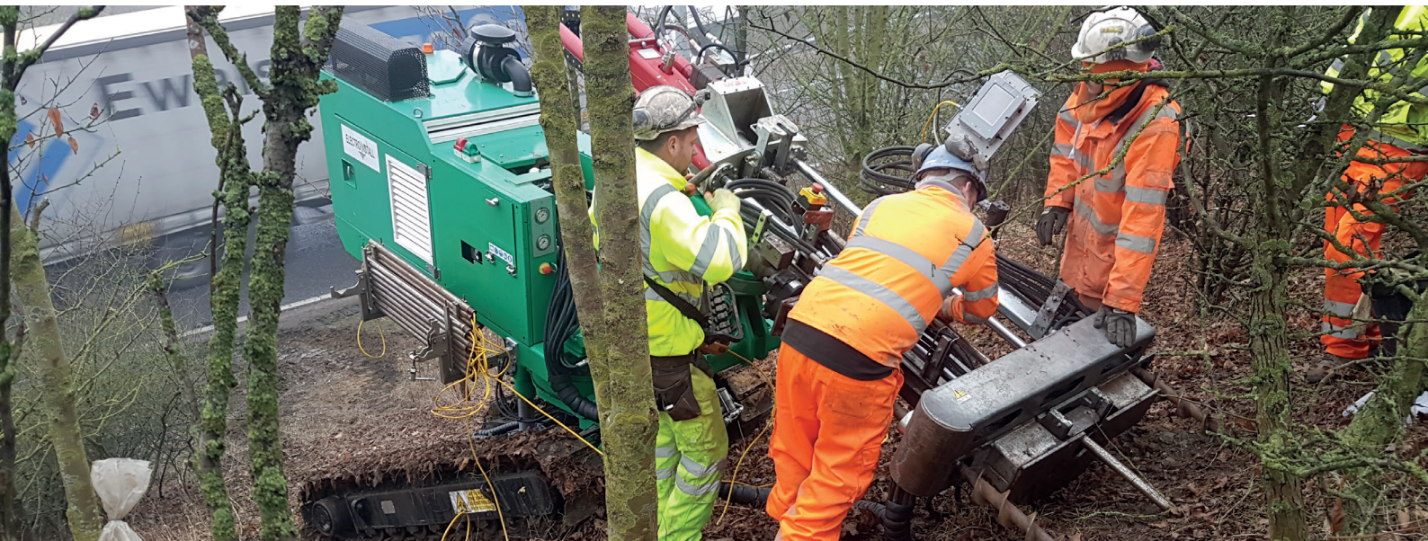
Unique Worldwide CPTu Slope climbing rig, remote control, self-levelling, drill at any angle. GI for proposed Electrokinetic remediation. Photo: A14 Brampton Hut, Amey/Highways England, 2017
