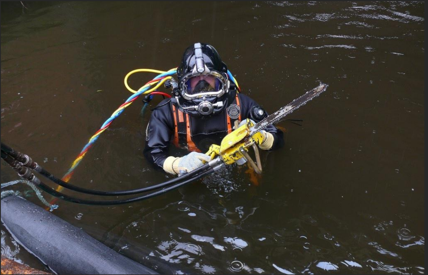
Once it was safe for the AquaticEngineering dive team to enter the water there were old wooden revetment piles to be removed below water.
