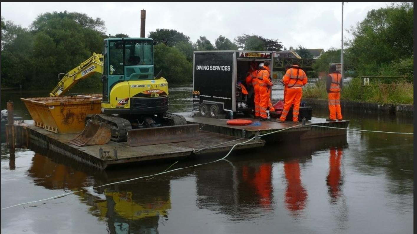
Silt around the bridge pier required removing and the riverbed reprofiling before the underwater grout mattresses could be installed and filled – these would also require being attached to stainless eye bolts which were drilled into the submerged pier.
