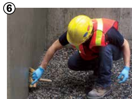
6 Waterproof where existing membranes have failed or where there was no initial waterproofing with Krystol T1 & T2®; a cementitious slurry system that becomes an integral part of the concrete to prevent water ingress.
