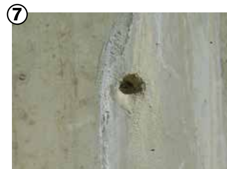
7 Repair leaking pipe penetrations and tie holes with Krystol Leak Repair System.
