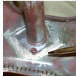
Pyro-Putty® 653 seals corroded burner manifold.
